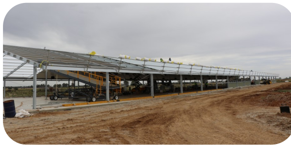
TOP: Council Chief Executive Officer, Geoff Rollinson (left), Mayor Garner Smith and construction manager, Craig Lord tour one of the sheds at the Kinross Farms Kerang East site. ABOVE: Construction of the Kinross Farms' large-scale free-range egg project at Kerang East is on track to be operational by June.
